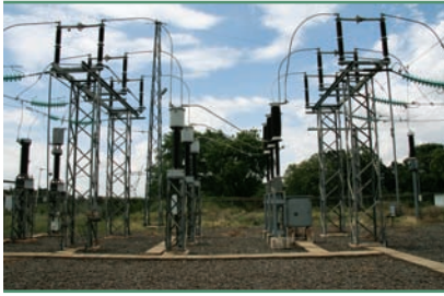
Kilimanjaro-Arusha Transmission Line Project in Tanzania co-financed with the World Bank
