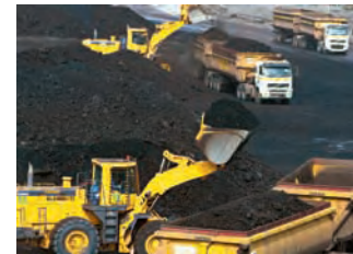
Road trains await their cargo of coal before embarking upon 75km journey along haul road to Kelanis River Terminal.
