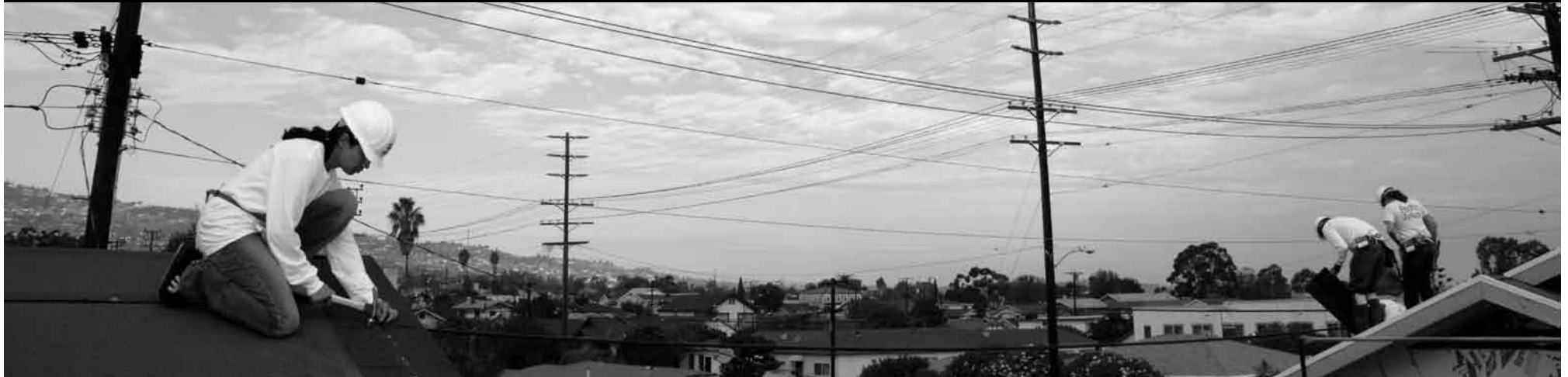
USA: On the roof of a multi-family housing project in Los Angeles during Jimmy Carter Work Project 2007.
