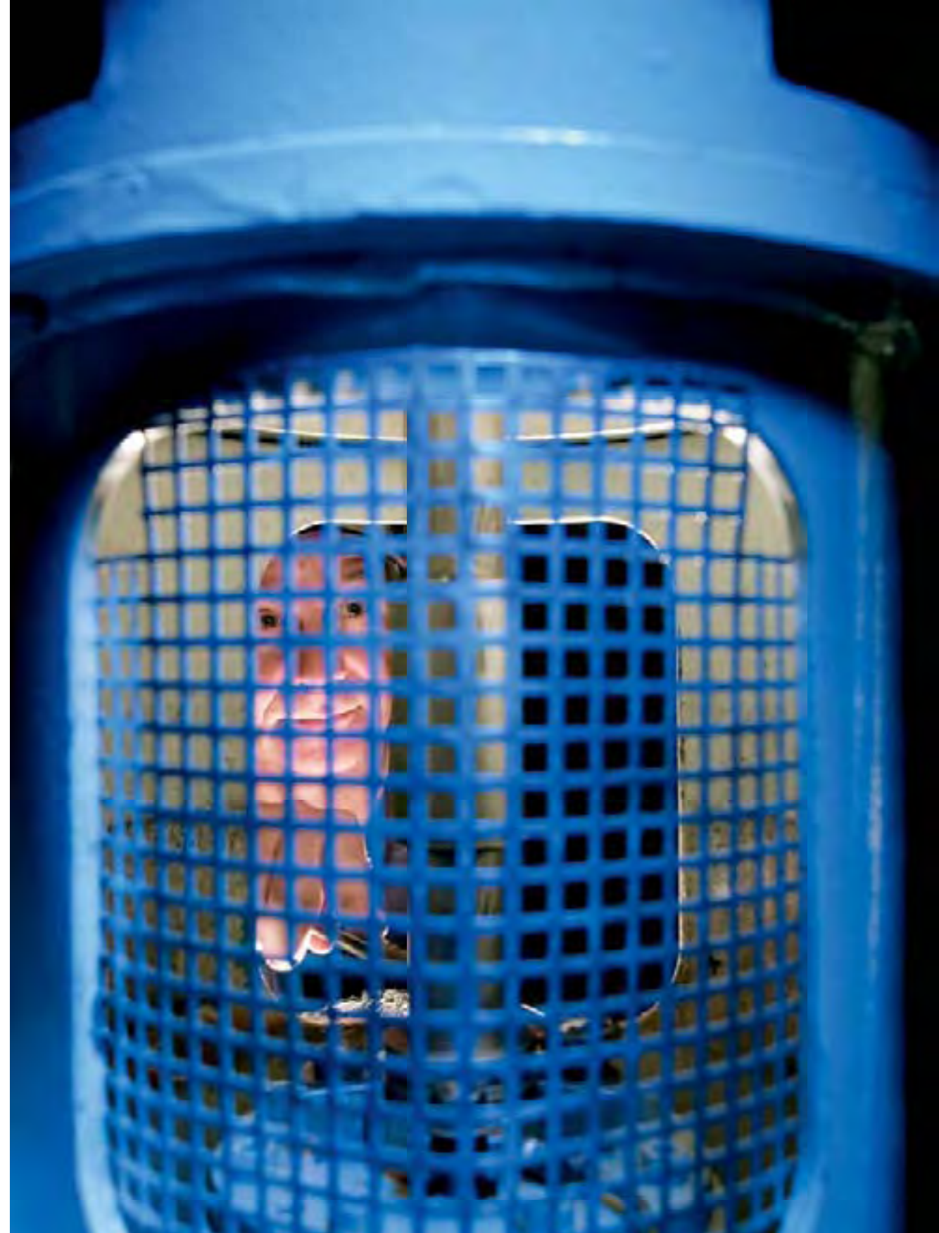
Treatment Plant Operator Dan Prinvale adjusts the packing on a vertical turbine water pump. This type of maintenance prolongs the life of our equipment, increasing our efficiency and enabling us to provide a reliable water supply to our customers.
