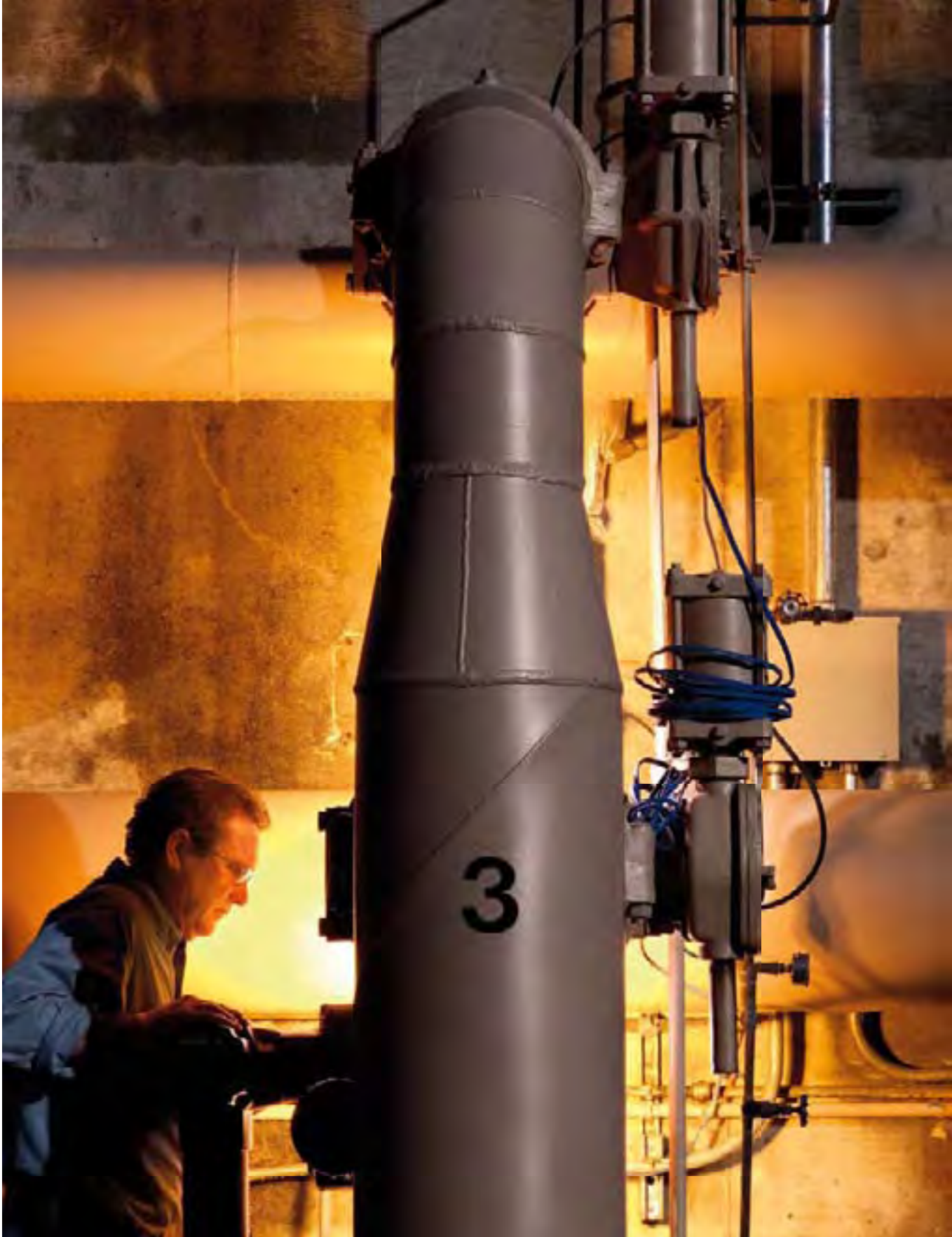
Treatment Plant Operator Bob Porter calibrates the new automatic controls on an ultraviolet treatment and filtration plant. At this plant, ultraviolet light treatment is an added safeguard to protect customers and ensure that the surface water treated here meets rigorous water quality standards.
