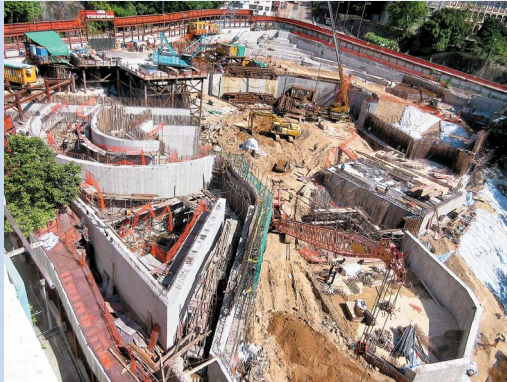
Redevelopment of Ming Wah Dai Ha underway 明華大廈重建工程進展順利
