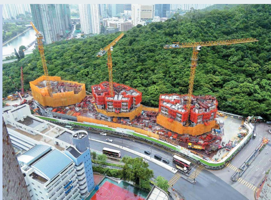
Superstructure works for Greenhill Villa in progress 「綠怡雅苑」正進行上蓋工程
