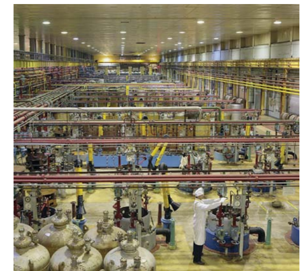
Condensing evaporating plants (JSC "SCC")
