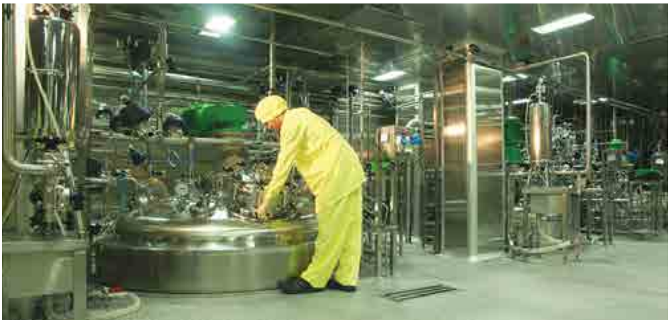
Inside of a Vaccine production plant
