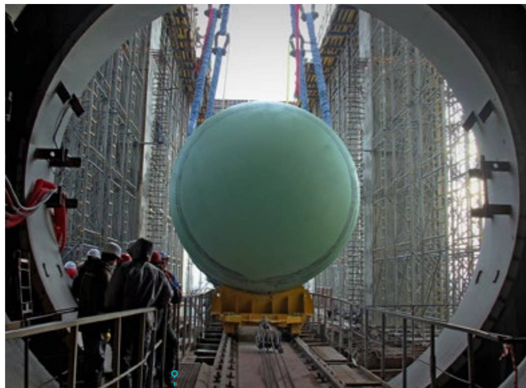
The reactor pressure vessel of Power Unit No. 2 of Belarus NPP was installed
