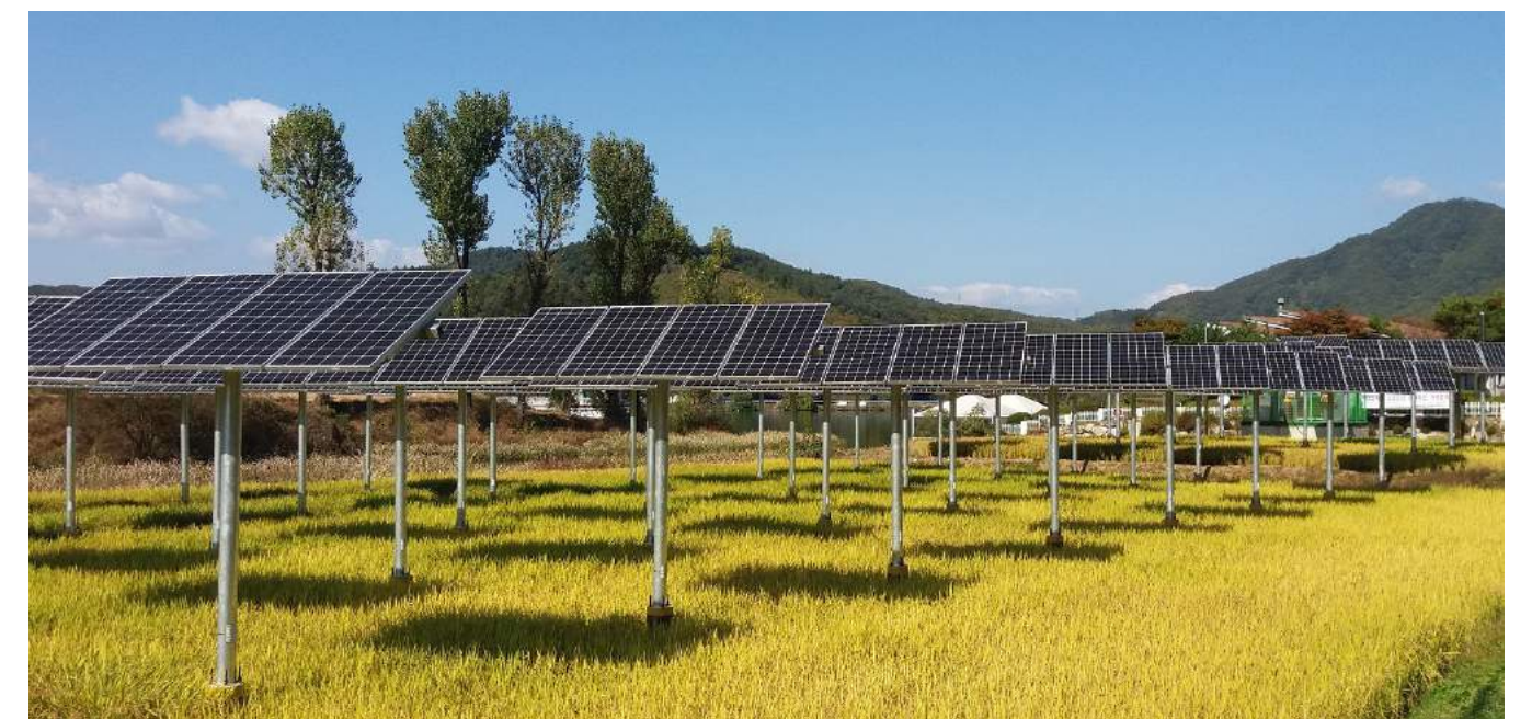
▲ Grid-connected solar photovoltaic power generating system in agricultural management
