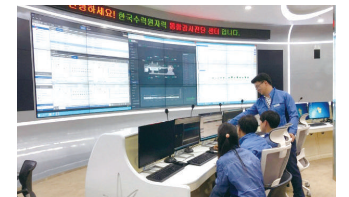
▲ Automatic facility failure prediction and diagnosis system
