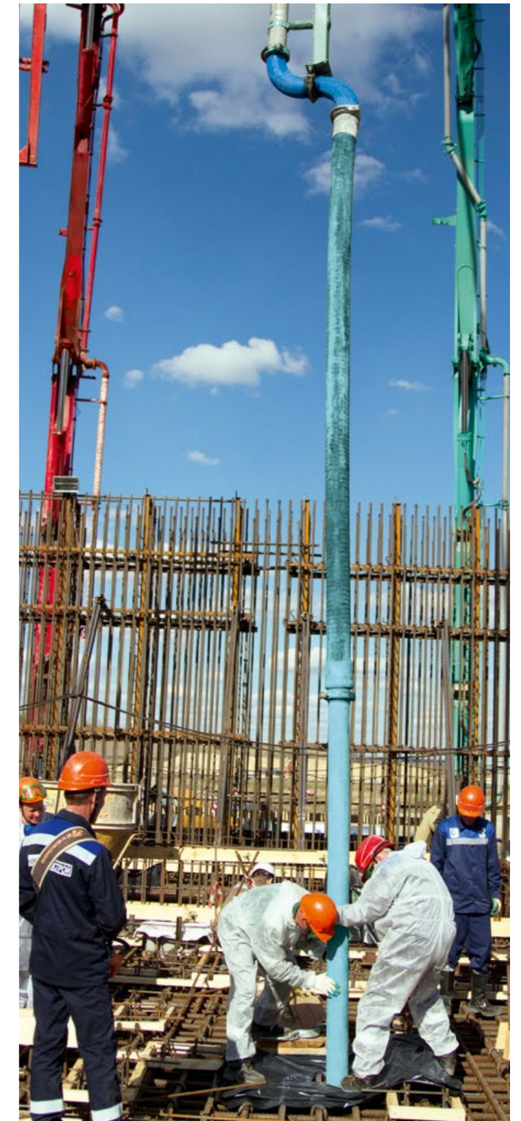
Start of the foundation slab concreting in the reactor building at Kursk NPP-2 Unit 1 (Russia)
